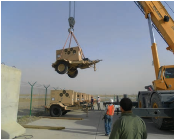
AMMPS units being readied for fielding to Afghanistan.
