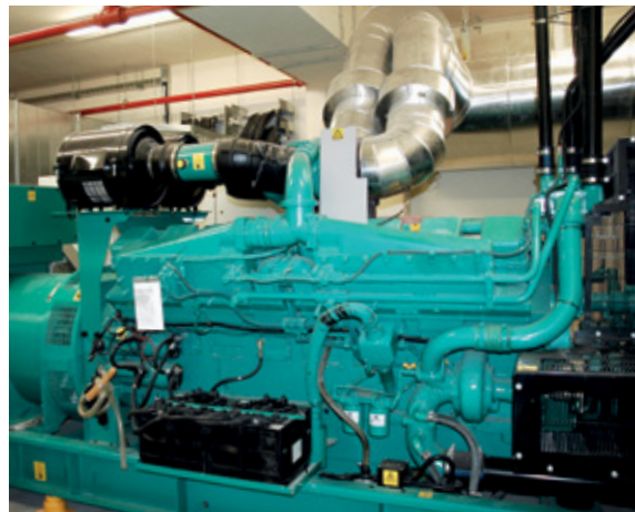
One of two Cummins Power Generation C1675 D5A generator sets
