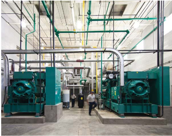
A pair of 1,750 kWe Cummins C1750 N6C generator sets run on either biogas or pipeline natural gas as required
