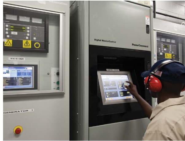
Cummins switchgear allows the system to deliver both base-load renewable cogeneration and island-mode "emergency" power
