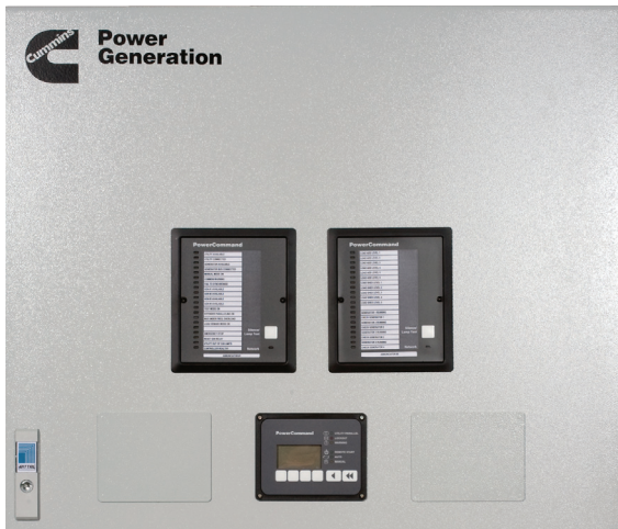
A DMC 1000 Load Management Panel controls four Cummins Power Generation generator sets
