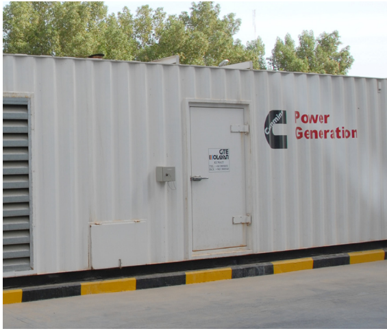
The HQ installation benefits from a sound attenuated container
