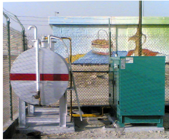
Zain has generator sets installed at around 300 locations
